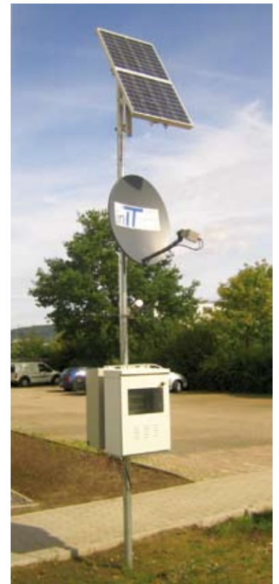
Energieautarke Messbake für Live-Messungen in Satelliten- und Mobilfunknetzen Energy self-sufficient station pole for live measurements in satellite and cellular networks
